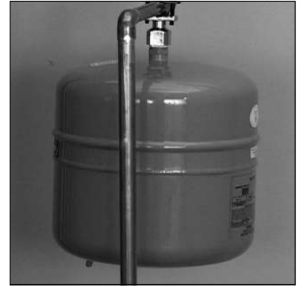
Figure 19 - The Thermal Expansion Tank should be pressurized with air, to match the home's incoming water pressure.
