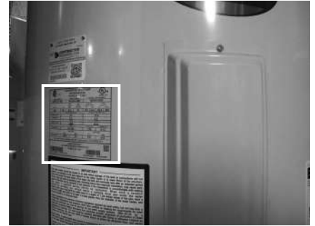
Figure 22 - The water heater’s electrical requirements can be determined from the data plate.
